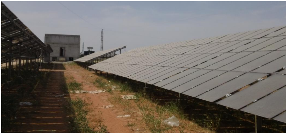
5.5 MW Solar Power Plant at Tinvari, Rajasthan
