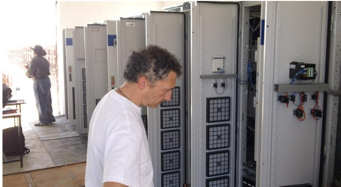
VTI Engineers at an Inverter room Tinvari, Rajasthan
