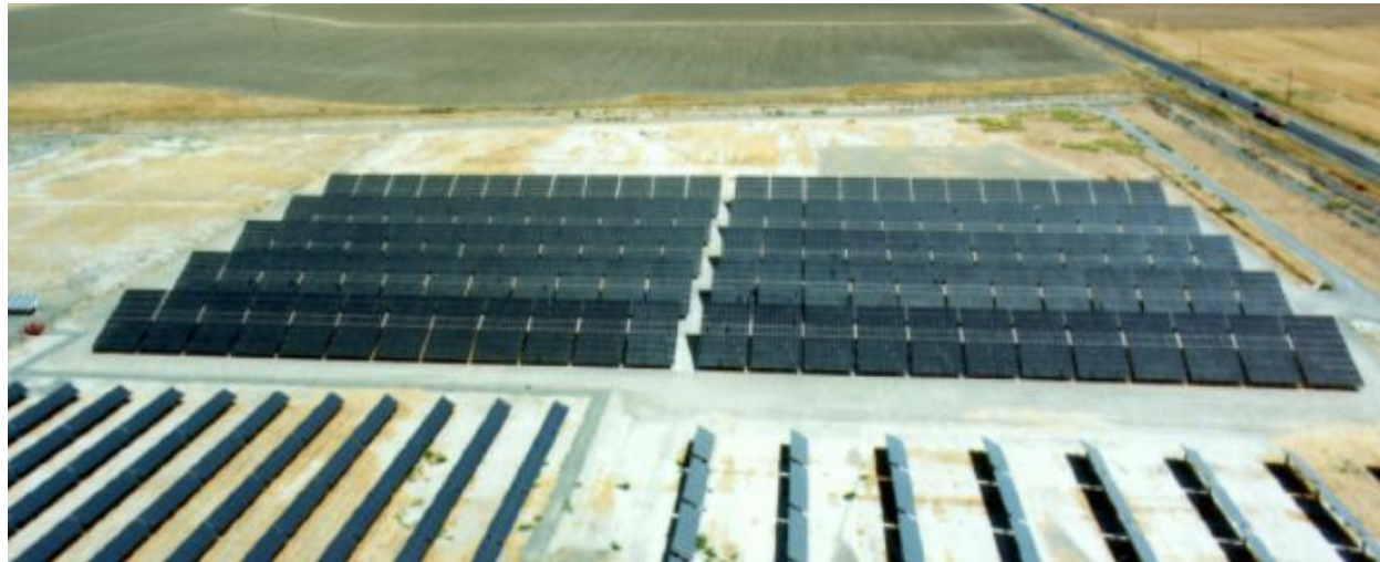
400kW Solar Power Plant; Boron, California
