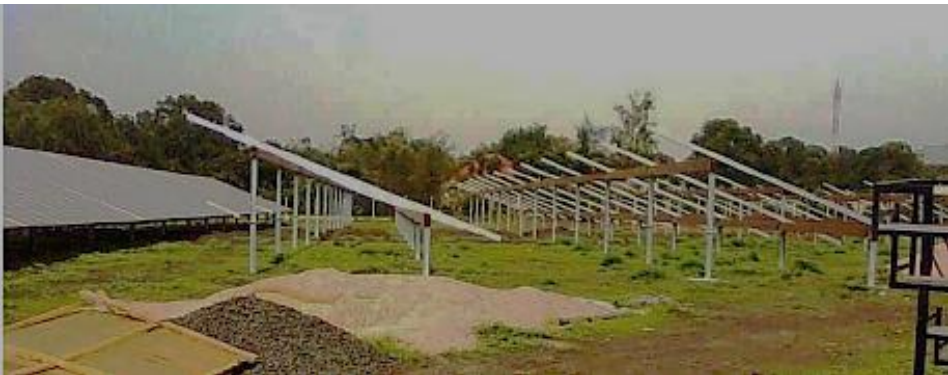
DPSC Ltd., 2MW Solar Power Plant Asansol, India
